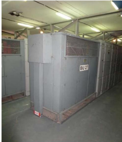
Figure 1.14 Transformer Component located at Zaporizhzhia Nuclear Power Plant (NPP)
