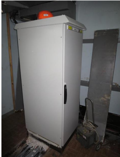
Figure 1.16 Control Monitor Cabinet located at Zaporizhzhia Nuclear Power Plant (NPP)
